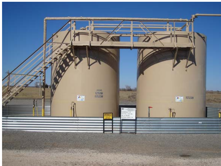
Figure 1: Typical Tank Battery
